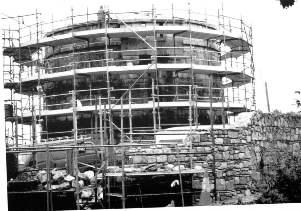
Tower during restoration – viewed from Killiney Hill Road As part of the extensive renovations the tower had to be repointed and some elements replaced. The perimeter wall at the public roadway had to be repaired and the entrance moved. The scaffolding, shown here, was in place for 9 weeks.
